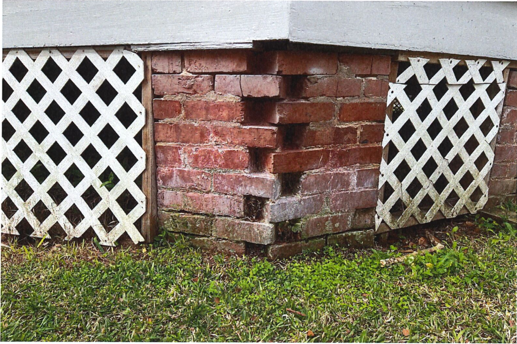
Eroded Pier - East
