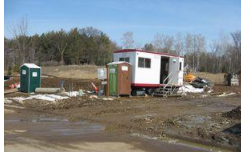
Example of a site with poor vehicle tracking practices.
