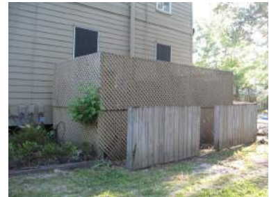
Appropriate screening of HVAC units at 22070 Highway 59.
