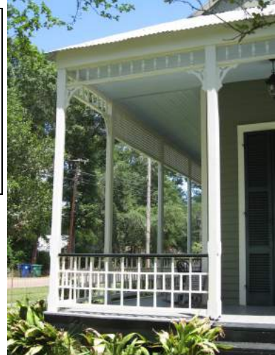
Porches are character-defining features in the historic district and original designs and features should be preserved and maintained (22222 Level Street).
