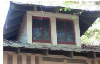
Roof features such as this hipped roof dormer at 71628 Leveson Street should not be removed or altered.
