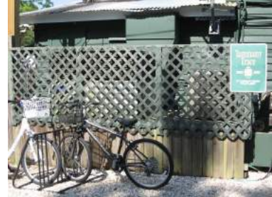
Lattice panels are used to screen the HVAC units at 22132 Level Street.
