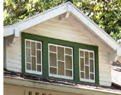
The original casement windows of this roof dormer help define the historic character of the dwelling (22014 2nd Street).
