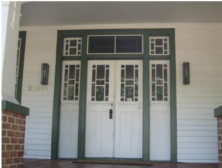
This entrance has its original multi-light double doors, sidelights, and transom (22014 2nd Street).
