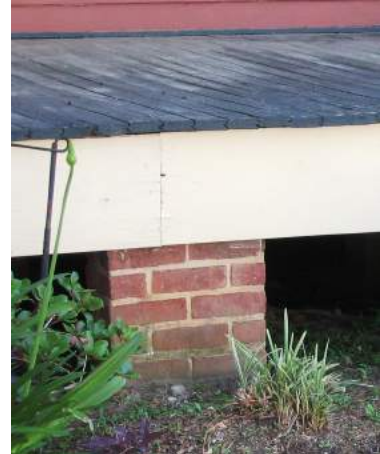
Many houses in the district have brick pier foundations that should be maintained and preserved (72104 Laurel Street).
