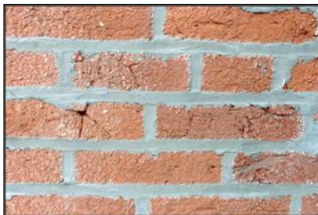
No—Do not repoint historic brick with hard mortars.
