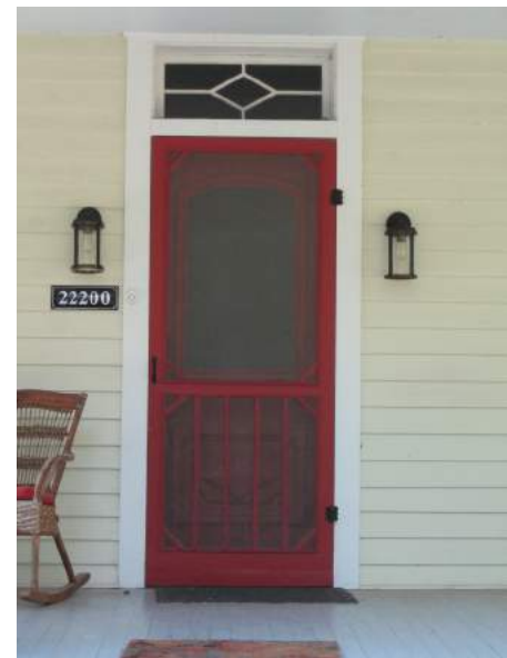
Appropriate screen door at 22200 Main Street.
