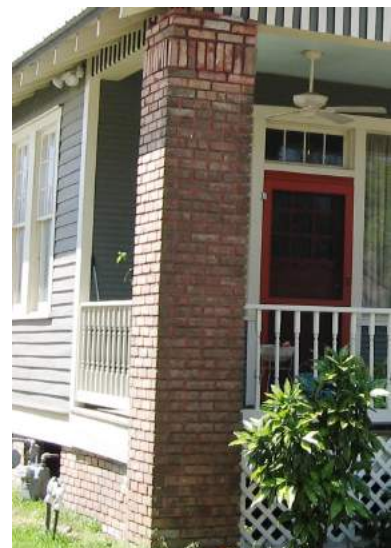
Brick is not a common wall surface in the district, but it is an important material for support features such as foundation and porch piers (22078 Main Street).
