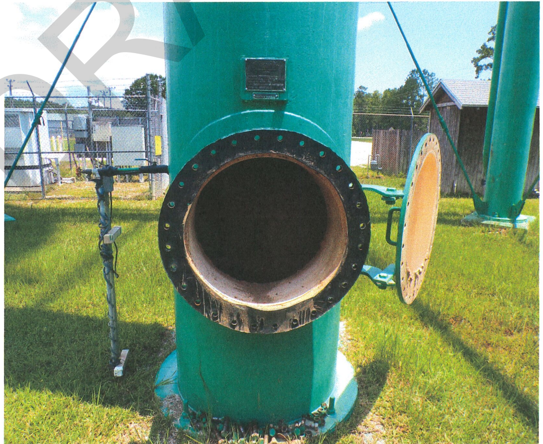
View of the riser manway. The manway has a 24" opening and is a bolted/flanged design.
