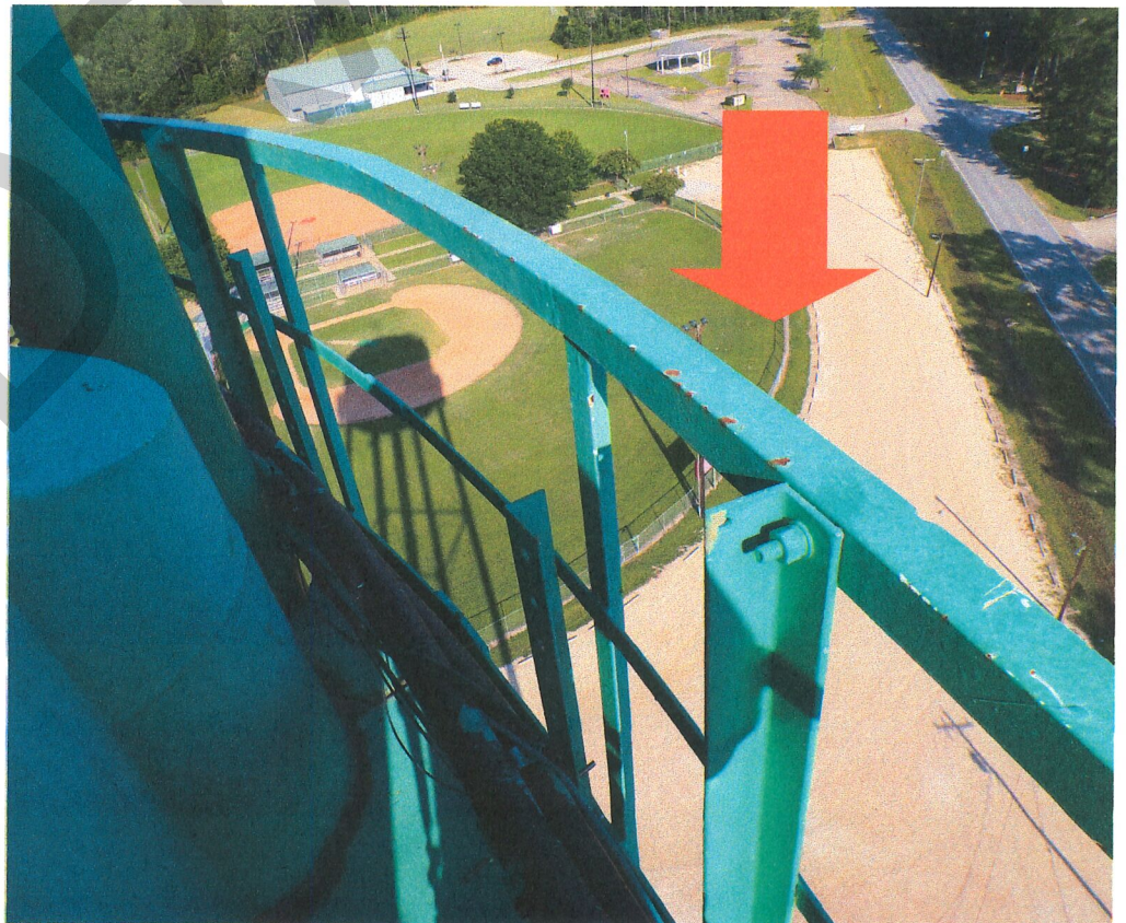
The coatings on the tank balcony hand-rail are in poor condition.
