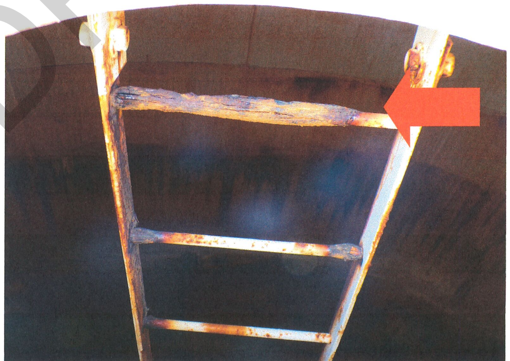
The interior ladder is in poor condition. Corrosion and coatings failure present. The ladder will need to be repaired at the time of the rehabilitation. No Safety cable system present.
