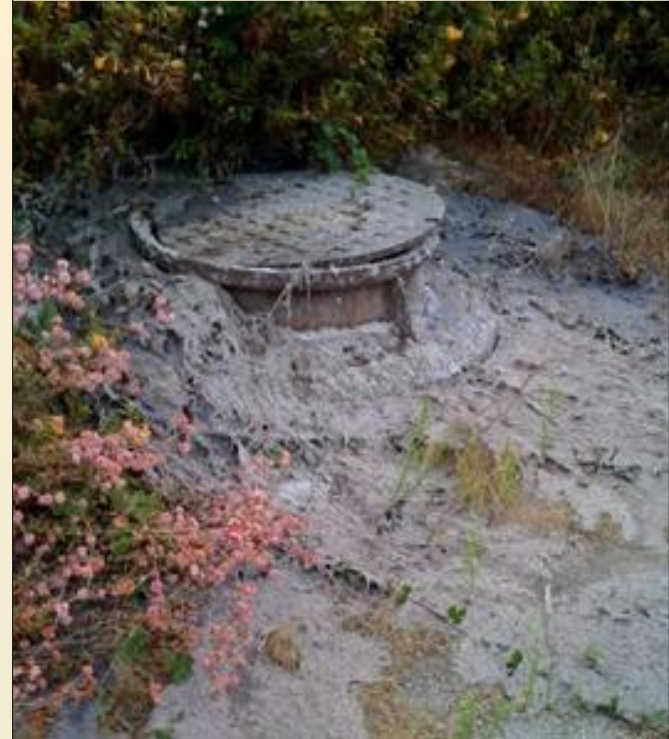
Above: Typical appearance of SSO at manhole
