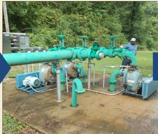
Pearl St. Lift Station
