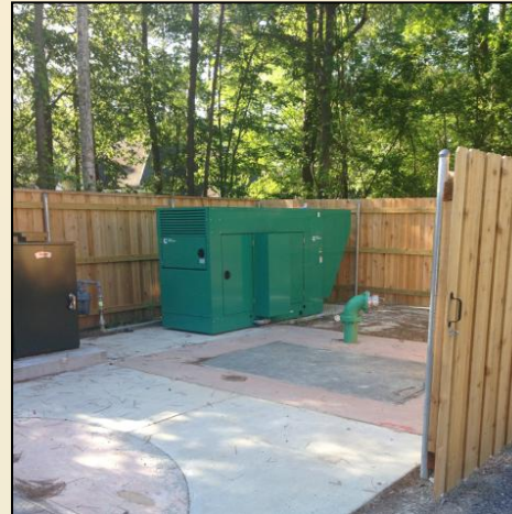
Left: CIPP & CCTV images Above: Standby generator at lift station
